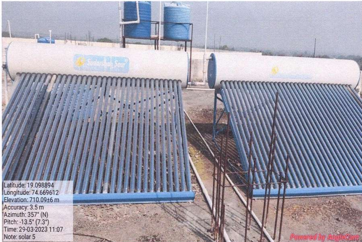
Image: Solar Water Heater
