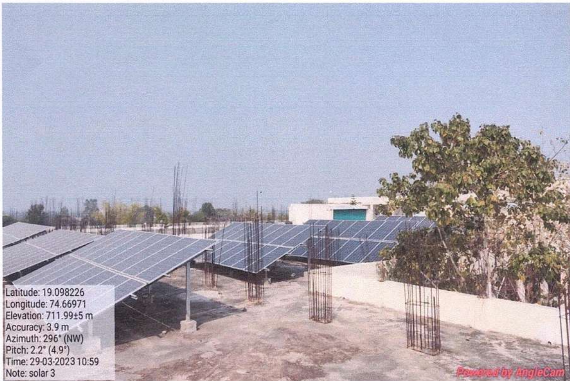
Image: PV Solar Plant
